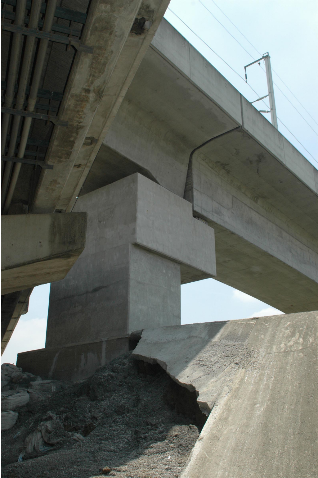
Figure 1.5 – Crumbling of embankment due to excessive vibration.
